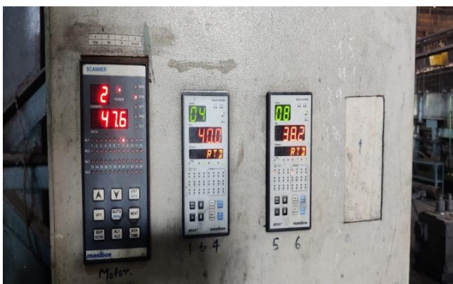
Fig. 5. PLC showing running temperature data .
