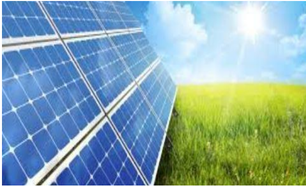
Fig. 4. A Photovoltaic Array
