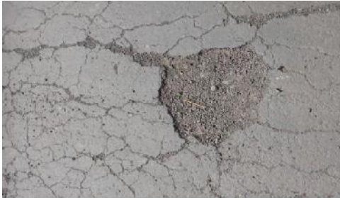
Fig. 1. Pothole on Asphalt Road
